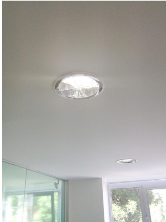
Figure 15: Garanti Bank Bilkent Branch Lighting (Image by Zeynep Dađlı, 2013)
